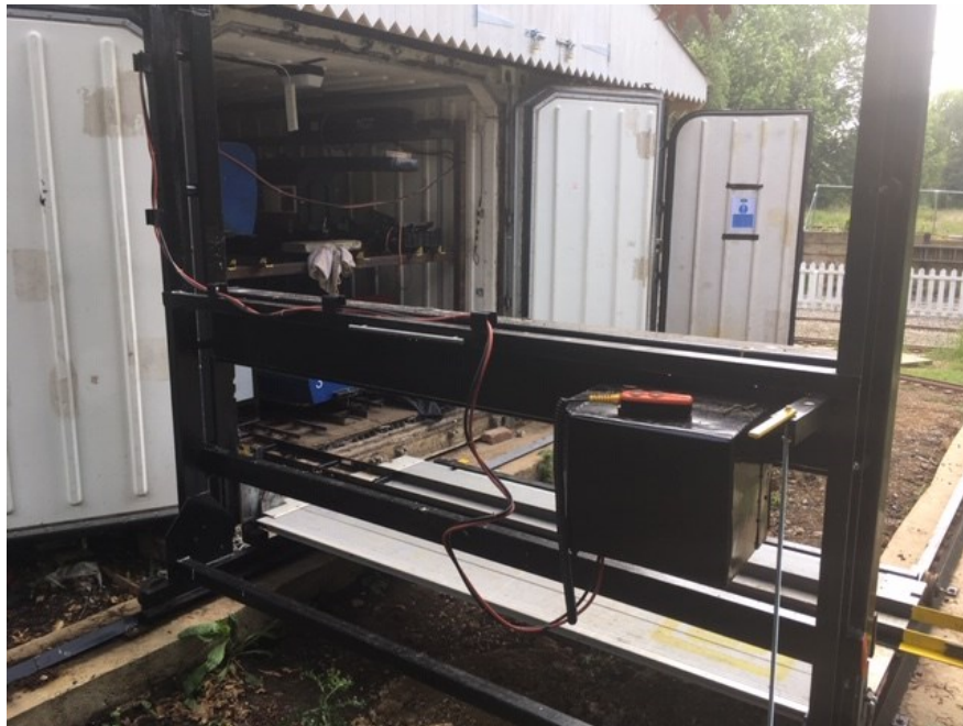
POWER AND CONTROL CABLE ARRANGEMENTS FROM CARRIAGE STORE ACROSS TRAVERSER FRAME AND INTO POWER PACK
